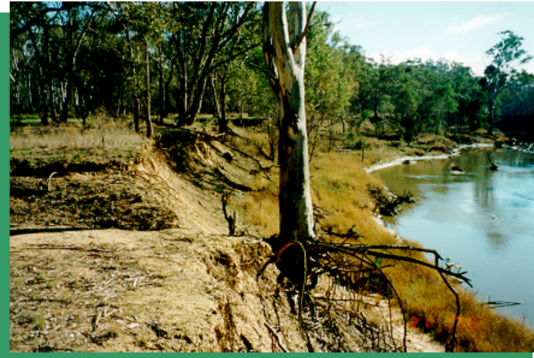
Figure 4b. River bank erosion and loss of riparian vegetation is severe in places.
