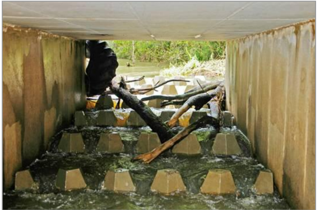
Figure 4. A box culvert with flow deflectors for enhancing passage of small fish. The debris was from a high flow event.
