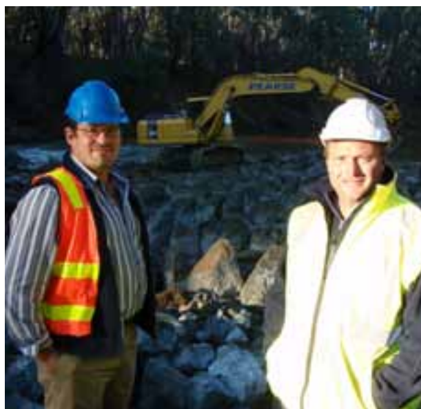
GB CMA's Carl Walters and Corey Wilson inspect works. Photo: Mark Turner, GB CMA
