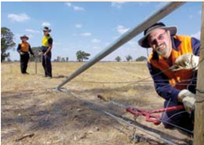
Above: Construction of revegetation plots on Murray River under the Drought Employment Program
