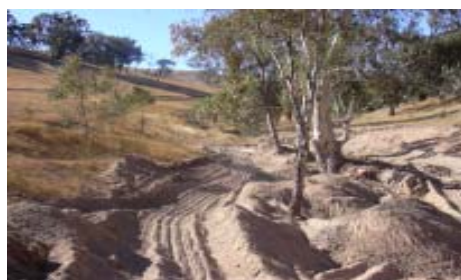
Unauthorised dam building works on a tributary of King Parrot Ck.
