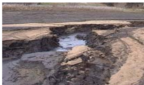
Erosion of sediments within the storage basin of the Honeysuckle Ck. Reservoir prior to decommissioning.
