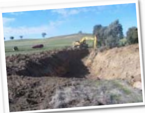
Preparation for installation of a rock chute to slow water velocity during peak flows - Bungeet.
